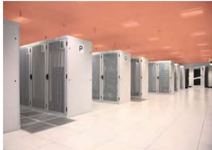
Ceiling protection at Data center
