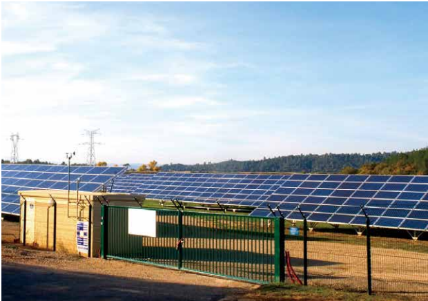
Perimeter protection X Laser scan / Photoelectric detectors
