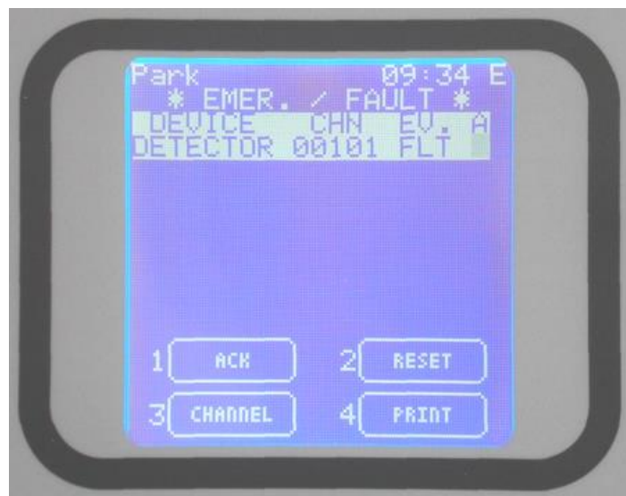
Fig. 3.5.1 c) Active events screen with fault only
