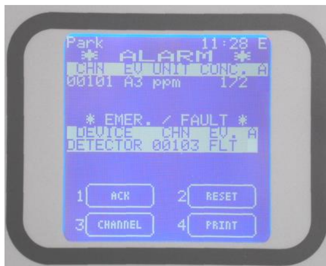
Fig. 3.5.1 a) Active Events screen with Alarm and Fault
