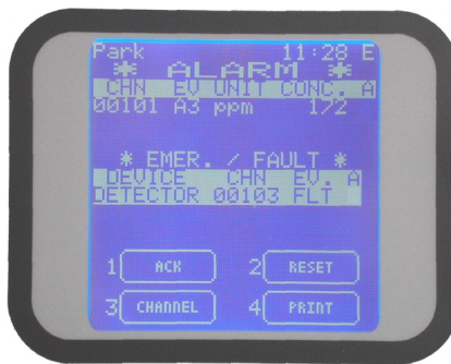
Figure 26) Active Events screen with Alarm and Fault
