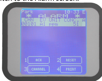
Figure 21) Typical ALARM state of the ACTIVE EVENTS screen.
