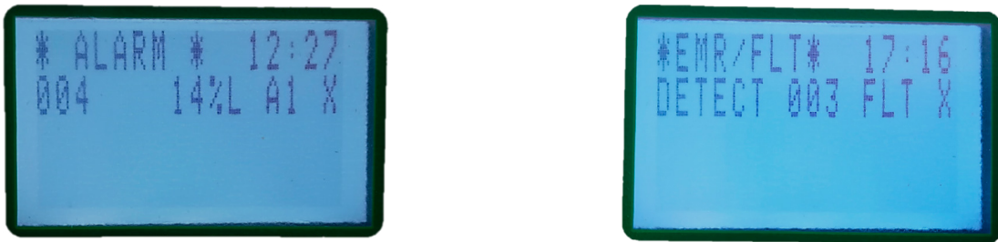
Figure 26) Active Events Screens: Alarm and Fault screen
