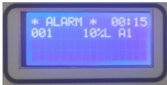
Fig. 3.2.1.b) Screen in Alarm status
