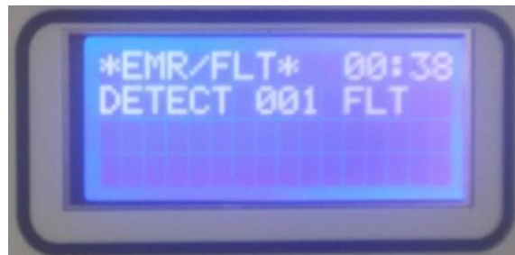
Fig. 3.2.1.d) Screen in Fault status
